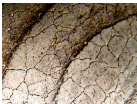
Figure 2: The reticulum of cracks on the tabla
